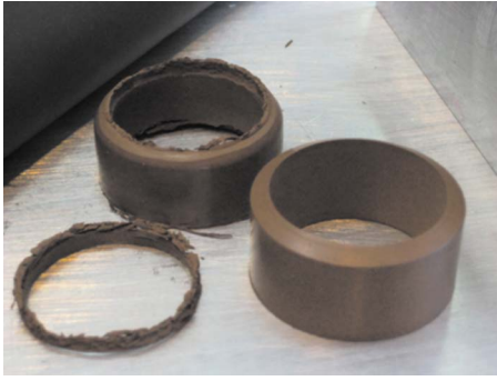
Fig. 15 Condition of Viton seal used in the probe connector before and after 28 days in rig
